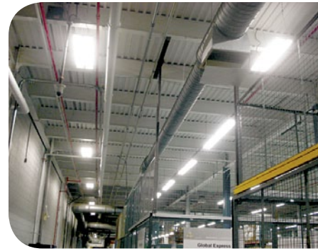
LIGHTING SYSTEM, TORONTO DOWNSVIEW FACILITY, CANADA
