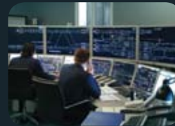
RAIL CONTROL SOLUTIONS CITYFLO mass transit signalling solutions including CBTC and INTERFLO mainline signalling solutions including ERTMS for onboard, wayside and control centre applications; EBI signalling product portfolio
